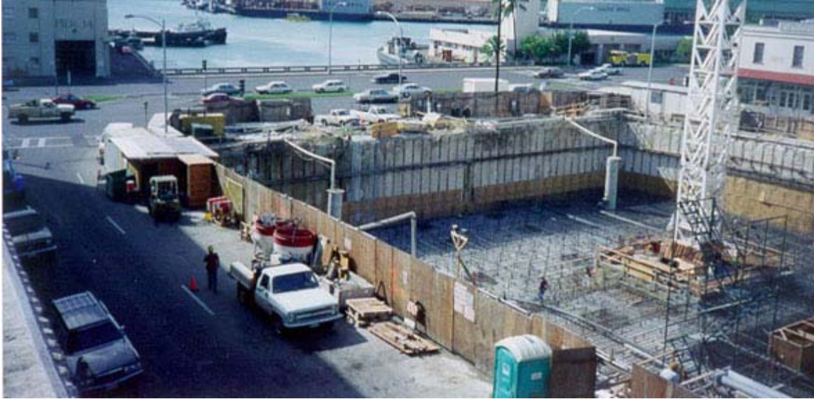
Figure 1 – 2. Marin Tower, Honolulu, HI Project Site (Picture from Schnabel Foundation Company, www.schnabel.com )
