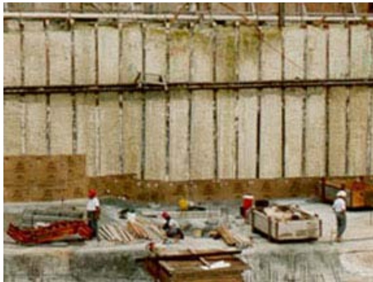
Figure 1 – 3. Marin Tower, Honolulu, HI Excavation Support System (Picture from Schnabel Foundation Company, www.schnabel.com )
