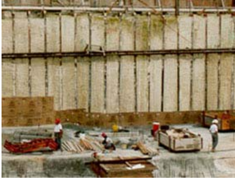
Figure 4 – 6. Marin Tower, Honolulu, HI Excavation Support System (Picture from Schnabel Foundation Company, www.schnabel.com )
